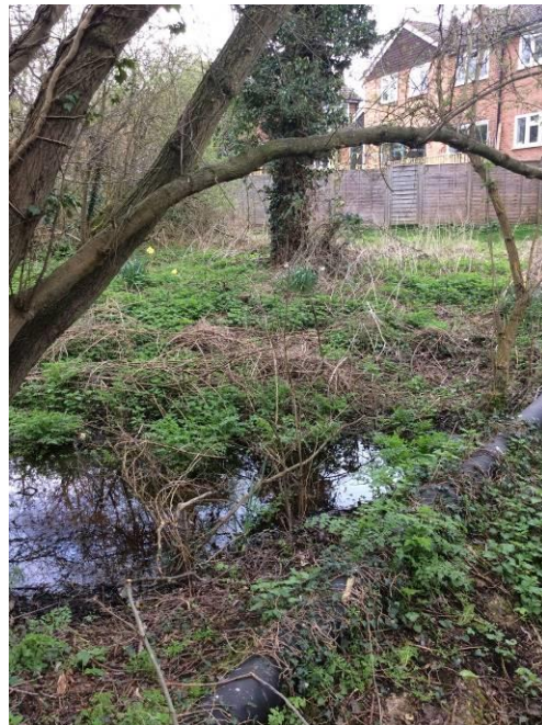
4. Raised foul pipe across paleo channel (TN3).
